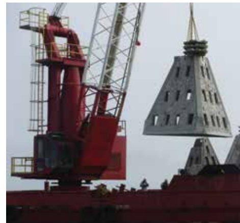
18 ft concrete module being deployed as artificial reefs in Gulf of Mexico approx 8 miles off Escambia County
