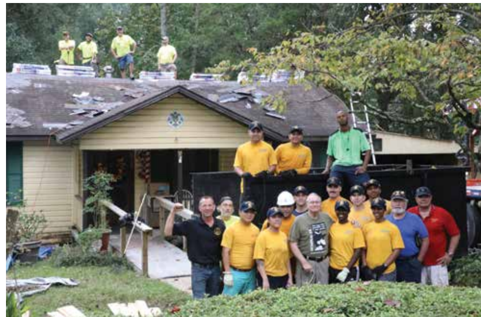
Guns to Hammers and AHERO join forces with the Cpl JR Spears Detachment of the Marine Corps League, Diamond Contractors, Merrill Land Construction and crew members of the U.S.S. Tripoli's crew to replace the dilapidated and leaking roof of Vietnam era Navy Corpsman, George "Doc" Dodge and his wife BeBe.
